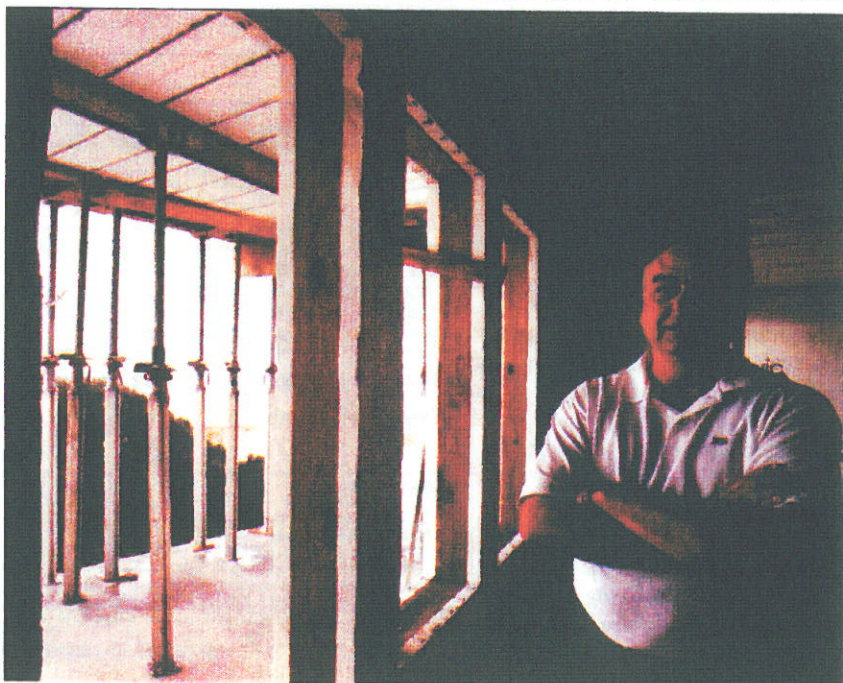
Architect Mike Piazza inspects the foam deck forms positioned atop ICF walls for the McMath home. Note the bracing for the cantilevered balconies.
